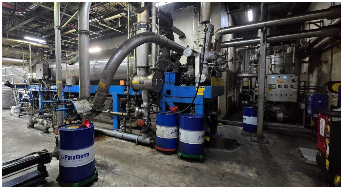
FIGURE 3-5: WILSONVILLE WWTP PADDLE DRYER
